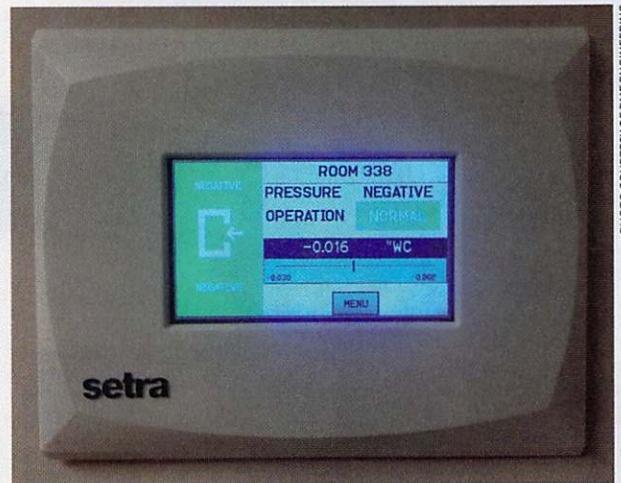
Typical space pressure monitor at the Medical University of South Carolina (MUSC).
