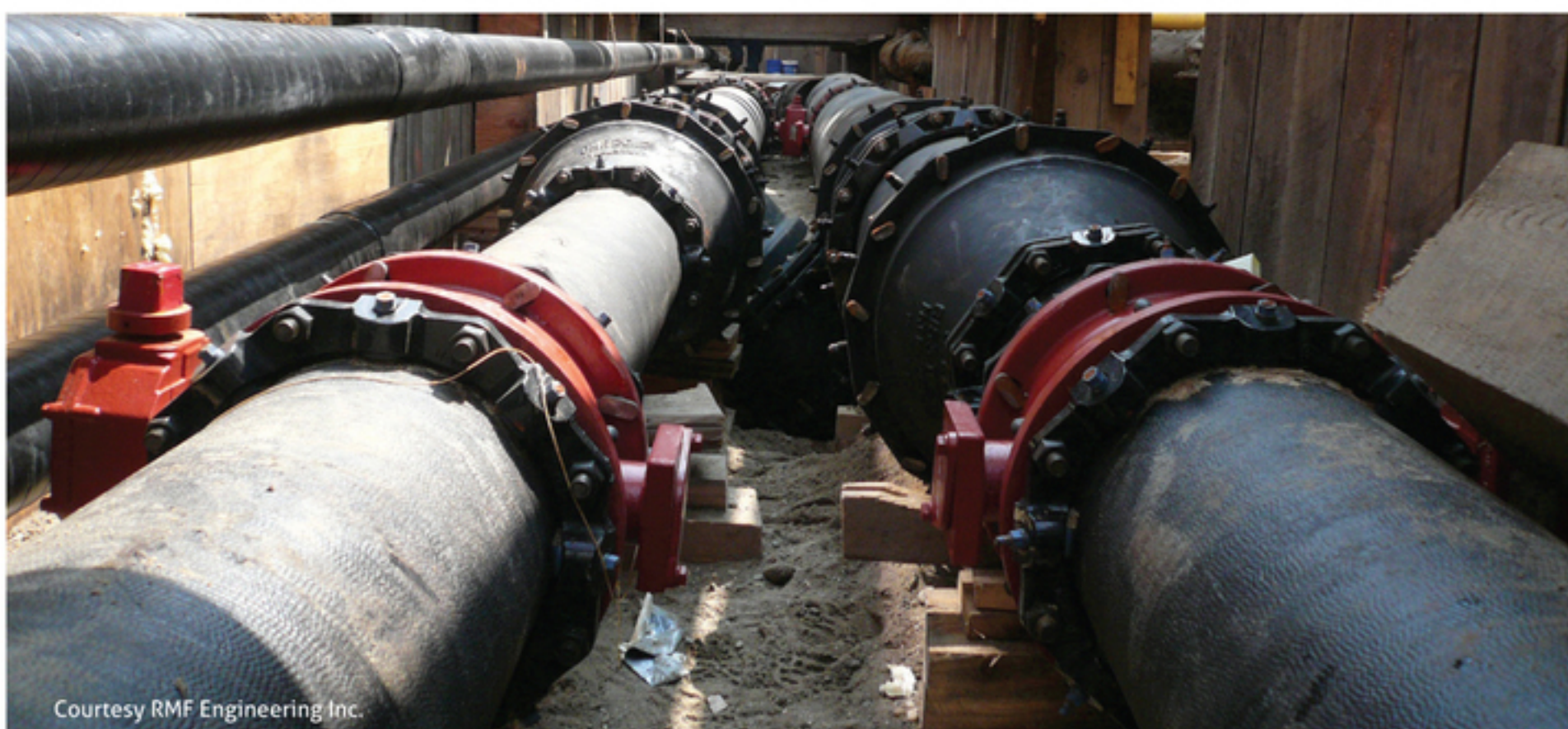
Renewal of Harvard University distribution systems typically requires keeping multiple services active during construction.
