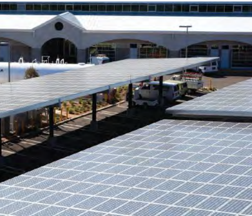
Figure 2: Energy efficiency goals are driving the need for renewable energy features (such as the solar panels in the photo), photovoltaic and solar hot water. Courtesy: Southland Engineering
