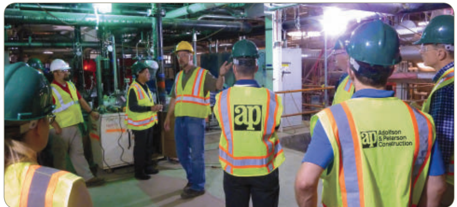
Conference attendees toured the ongoing construction of a state-of-the-art CHP facility: the University of Minnesota’s $96 million rehabilitation of the Old Main Heating Plant, built in 1912. The campus is targeting a 50 percent reduction in emissions by 2020 and carbon neutrality by 2050.
