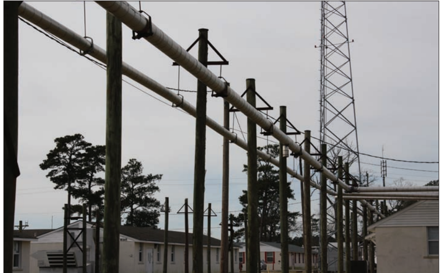
Marine Corps Base Camp Lejeune has multiple district steam utility systems including Hadnot Point, New River Air Station, Camp Johnson, Courthouse Bay, and Camp Geiger. Each location had been utilizing a central steam heating plant to generate and distribute high-pressure steam to over 500 buildings, with more than 50-mi of steam supply and condensate return piping. Above, pre-existing steam distribution at Camp Johnson, N.C. PHOTO COURTESY RMF ENGINEERING
