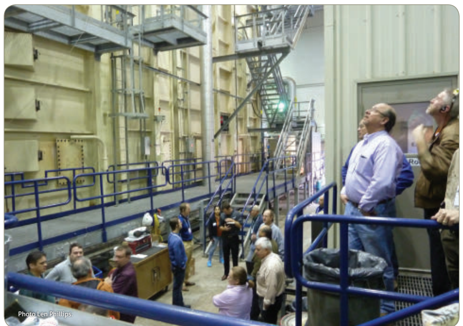
Conference goers touring the UT Austin district energy system were dwarfed by one of the plants’ heat recovery steam generators. The campus can island 100 percent, providing all of its electricity, heating and cooling demand at will.
